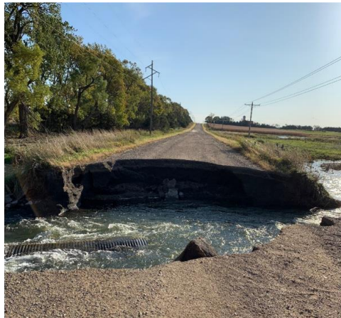
Figure 2. Work in water due to a road collapse may require US Army Corps of Engineers NWP or 401 or 404 depending on the method of repair. FEMA photo.
