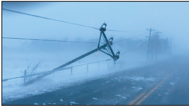
Overhead powerlines were torn down by a thick ice build-up combined with high winds during a blizzard that struck the state on Christmas Day 2016.
